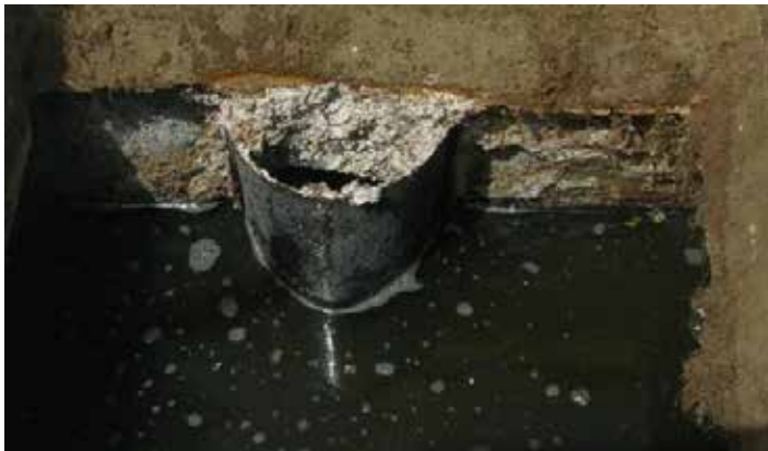
Photo 1 Concrete Corrosion around Outlet Baffle
