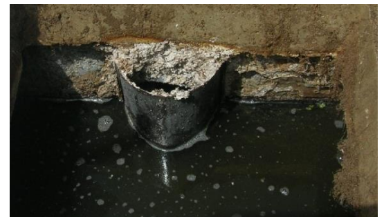
Illustration 1: Concrete Corrosion around Outlet Baffle
