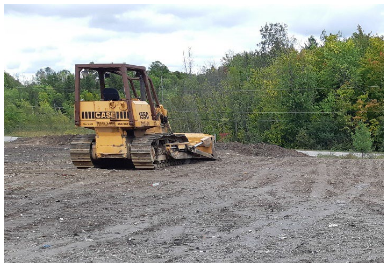
Figure 5 Garbage Compaction Equipment – Glen Tay WDS
