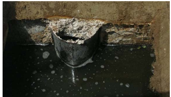
Illustration 1: Concrete Corrosion around Outlet Baffle
