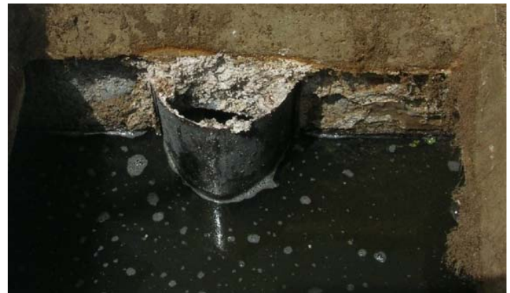
Illustration 1: Concrete Corrosion around Outlet Baffle
