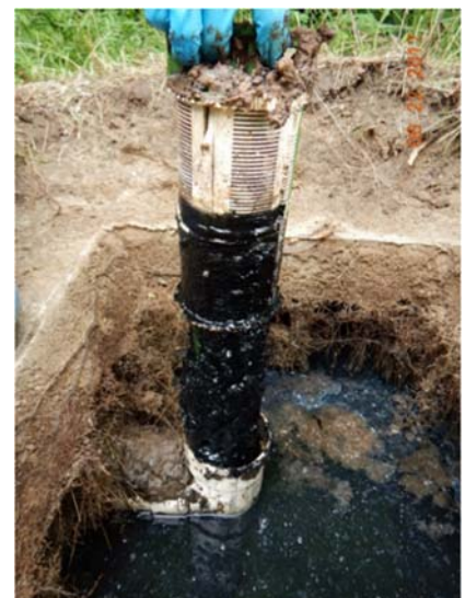
Illustration 2 – Clogged Effluent Filter
