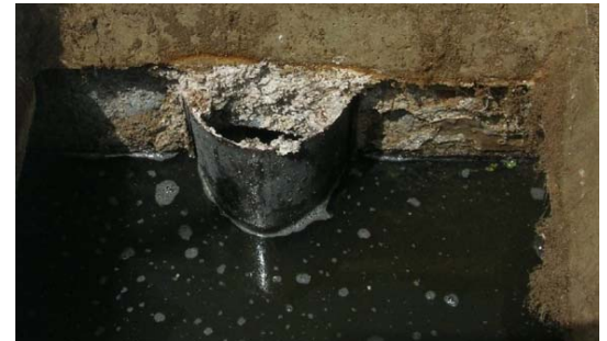
Illustration 1: Concrete Corrosion around Outlet Baffle
