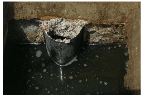
Illustration 1: Concrete Corrosion around Outlet Baffle
