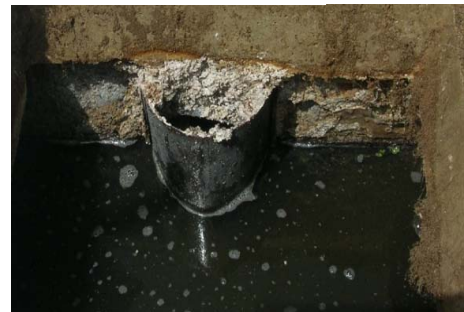
Illustration 1: Concrete Corrosion around Outlet Baffle
