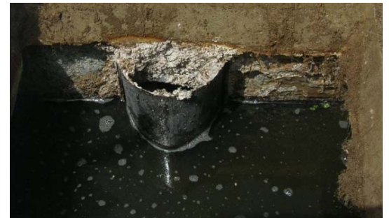
Illustration 1: Concrete Corrosion around Outlet Baffle
