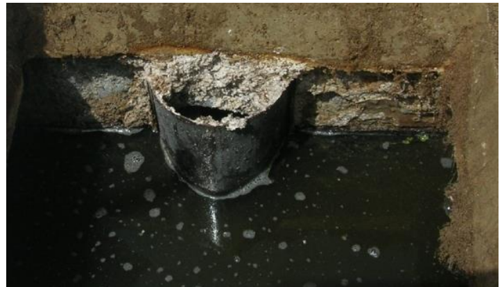
Illustration 1: Concrete Corrosion around Outlet Baffle
